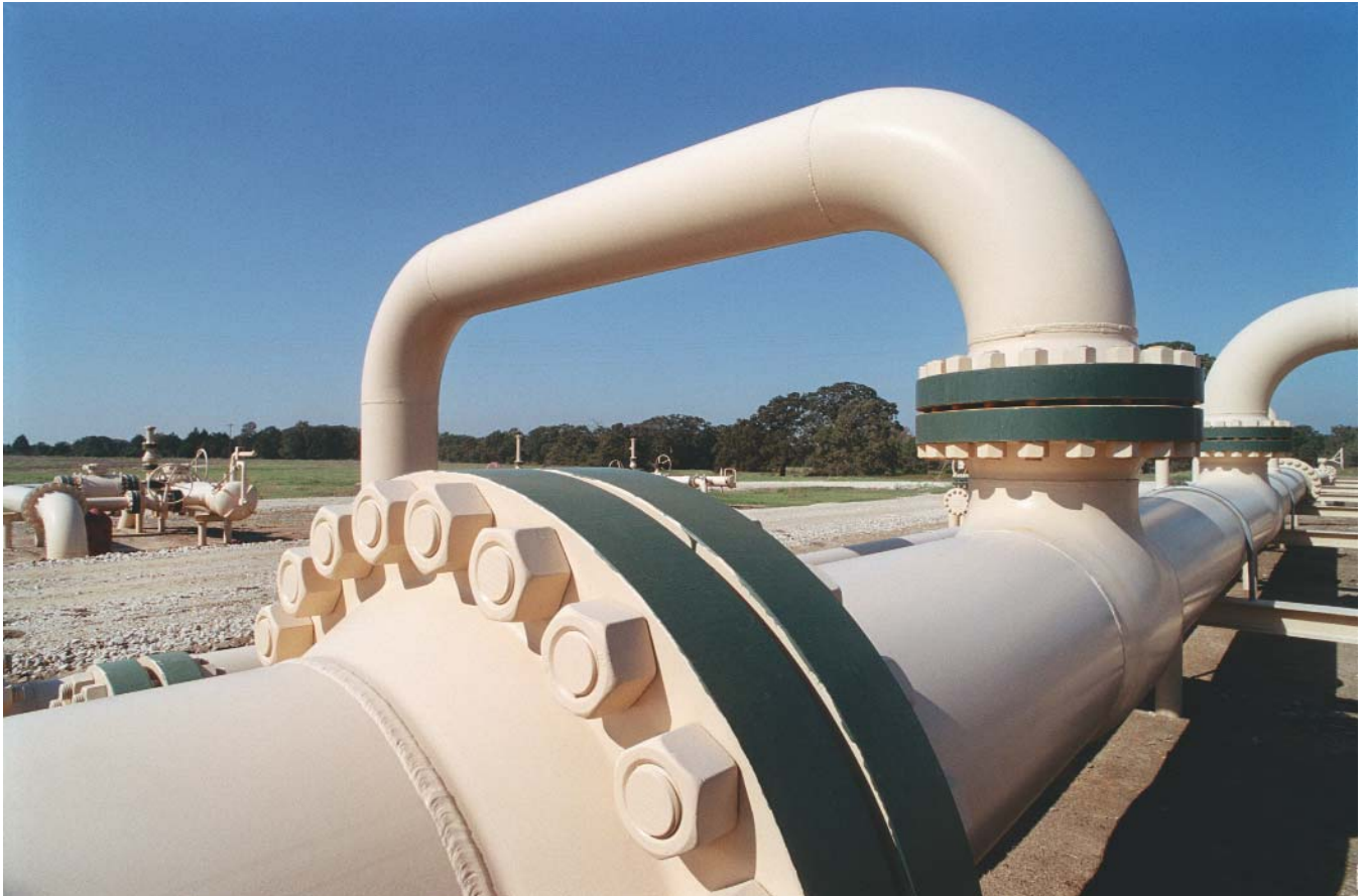
Compressor header for gas-gathering in the Freestone Trend. (Photo courtesy of XTO Energy Inc.)
